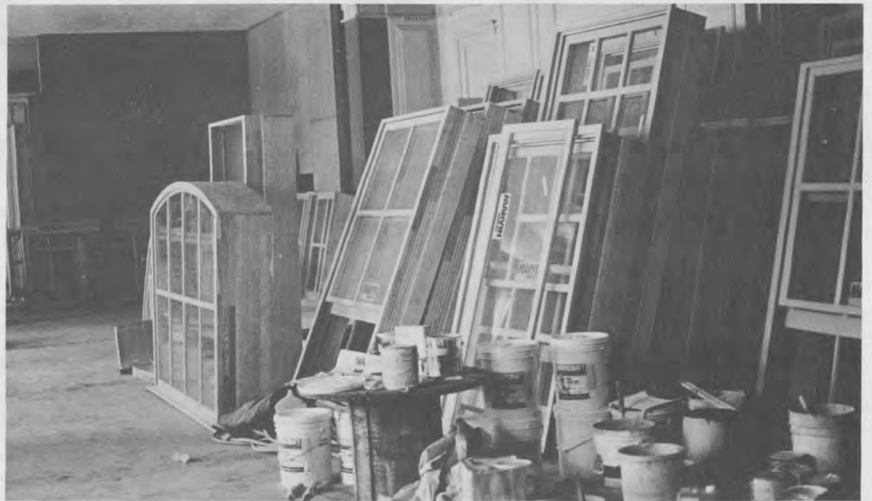
Windows wait in the lobby of the Memorial Building to be installed in the new fine arts wing.
